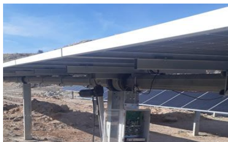
HB-DJ817T Electrical linkage, 10MW, 2024, Turkey
