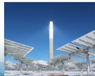
HBDJ816-Qinghai, 50MW, 2018, China
